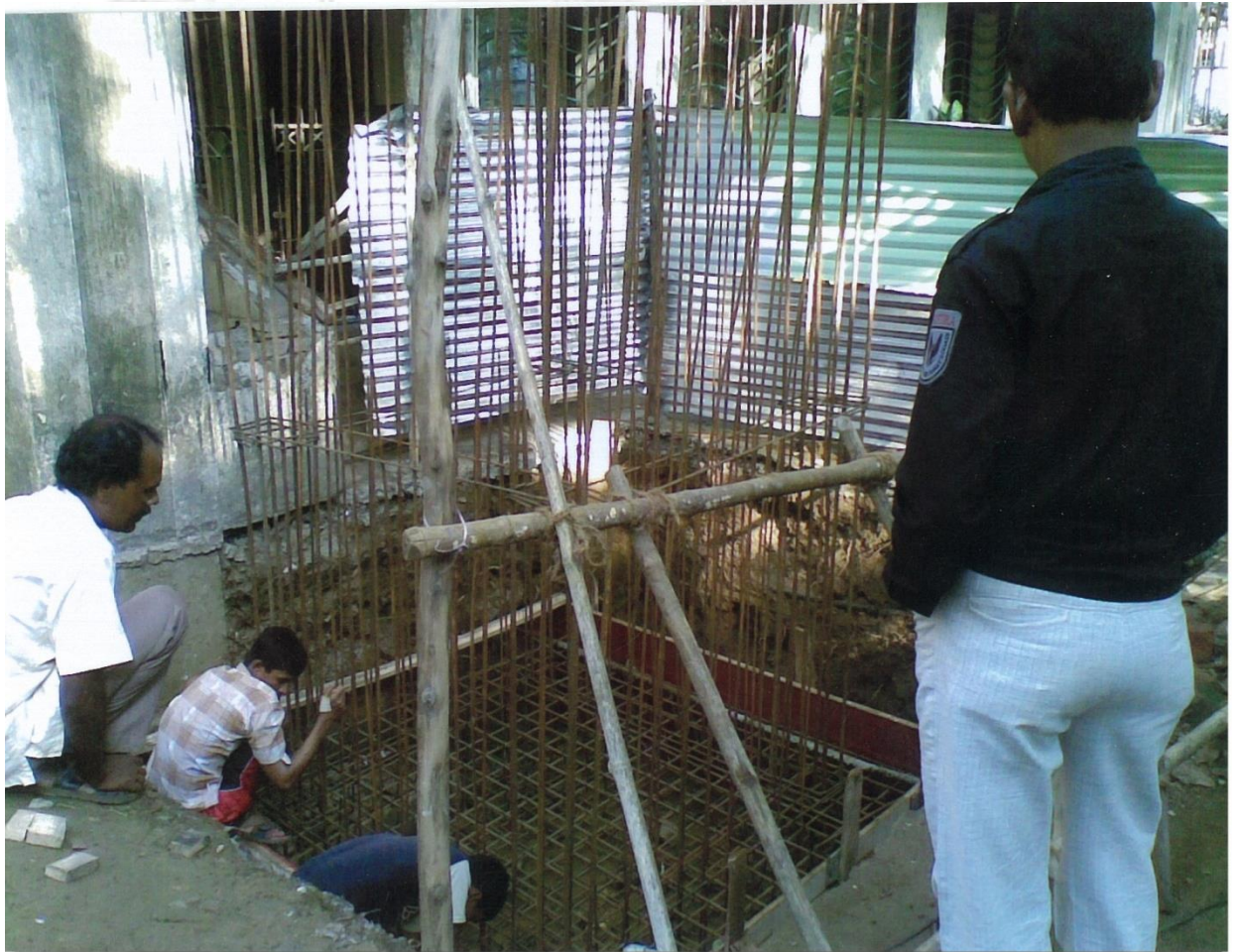
Shuttering work being done for the lift shaft Along with laying of steel
