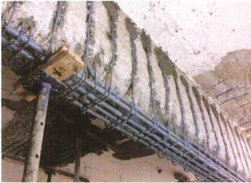
Cutting Loose Plaster & Loose Concrete & Applying Rustside & Bond Coat and new bar rings Epoxy Coat
