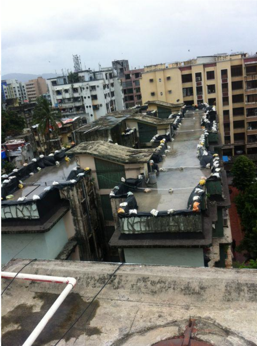
Terrace Waterproofing Ponding
